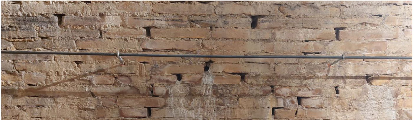
Holes for water collection
